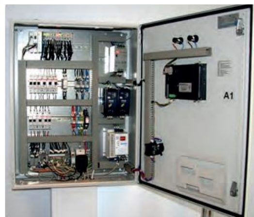
Fig. 21. Control system of the laboratory test rig
