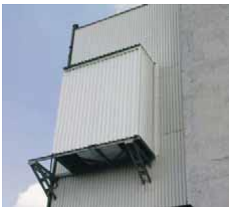
Fig. 18. Silencer of the air draw and ejector installed at the Jankowice Mine [17]
