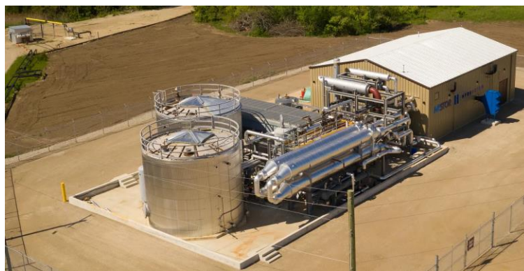
Fig. 10. A-CAES storage facility in Goderich, Ontario, Canada [16]
