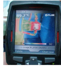
Fig. 27. Defective working pump
