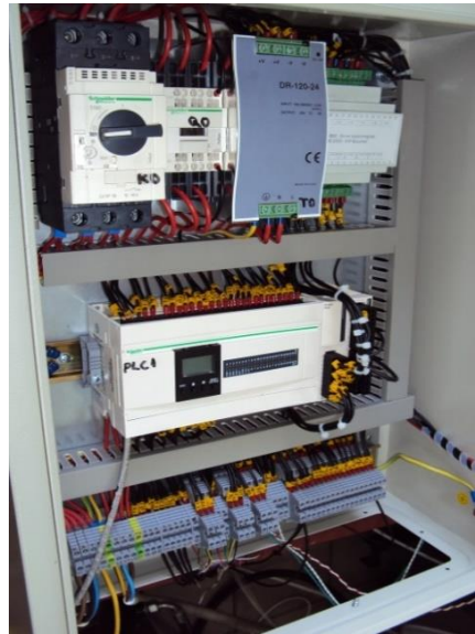
Fig.4. The electric panel
