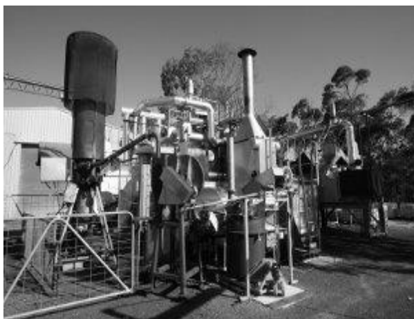
Fig. 4. Pyrolysis demonstrative plant manufactured by BEST Energies (USA)
