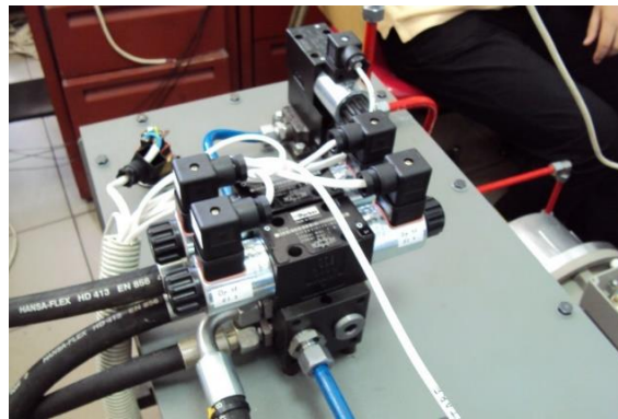
Fig.5. The proportional directional control valve
