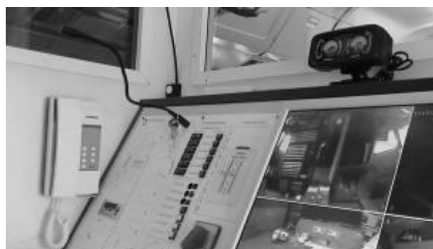
Fig.10. The control panel
